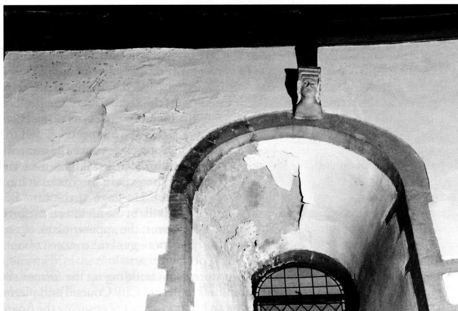
Fig. 10 St James's Priory, south aisle, detail showing damage caused by damp penetration Photograph, © English Heritage 2006
